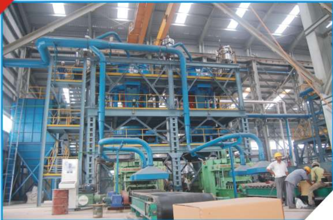
Taphole Clay Plant at Belpahar
